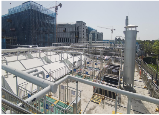
污水站加盖密封
